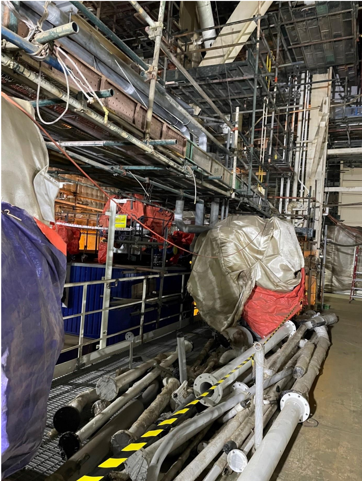
Figure 3-5 View inside the engine room
