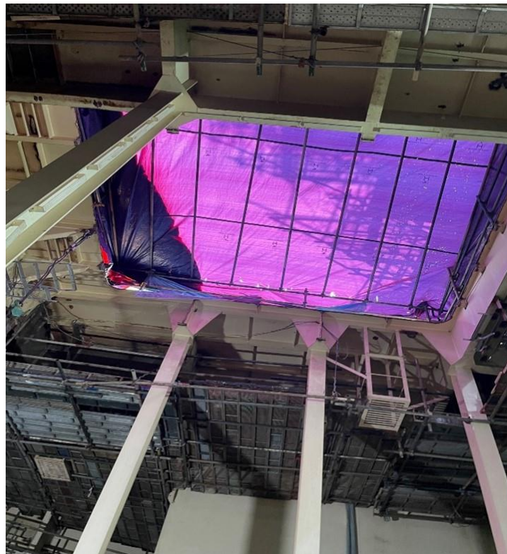
Figure 3-4 View inside the engine room showing the hole in the deck used to lower down all equipment and that will be closed in the coming days.
