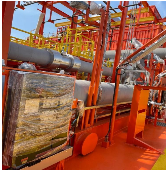
Figure 3-8 Metering skid piping
