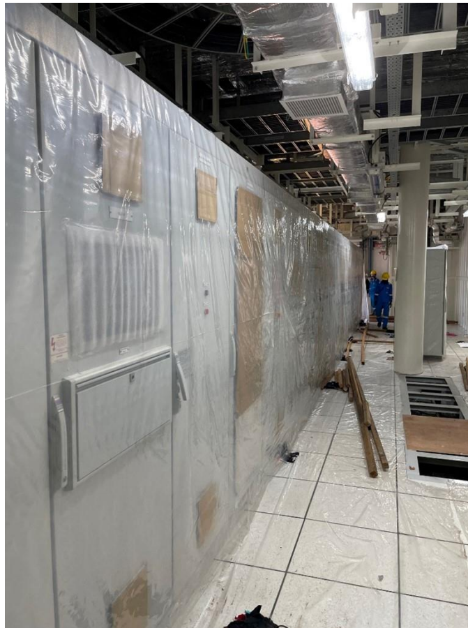
Figure 3-7 View inside the E-house
