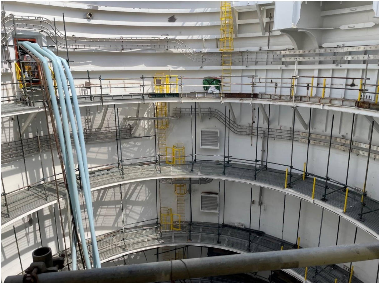
Figure 3-13 View inside the TMS
