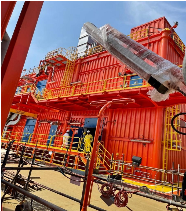
Figure 3-9 View of Module M60 -E-house
