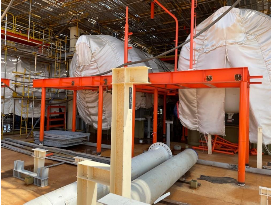
Figure 3-20 Inside view M30
